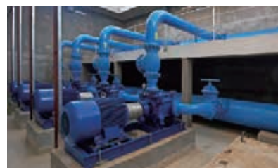
Building water pumps
