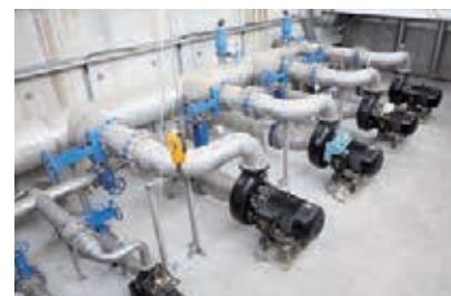
Sewage treatment plant
